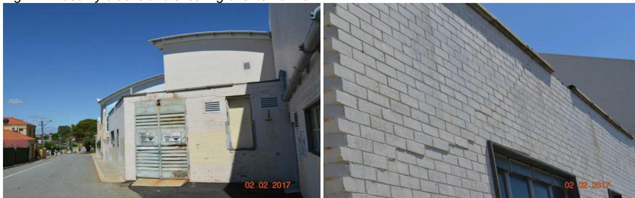
Fig. 1 – Masonry cracks and shearing of external wall
