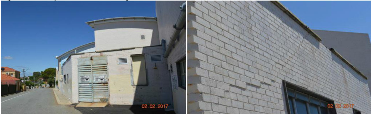
Fig. 1 – Masonry cracks and shearing of external wall
