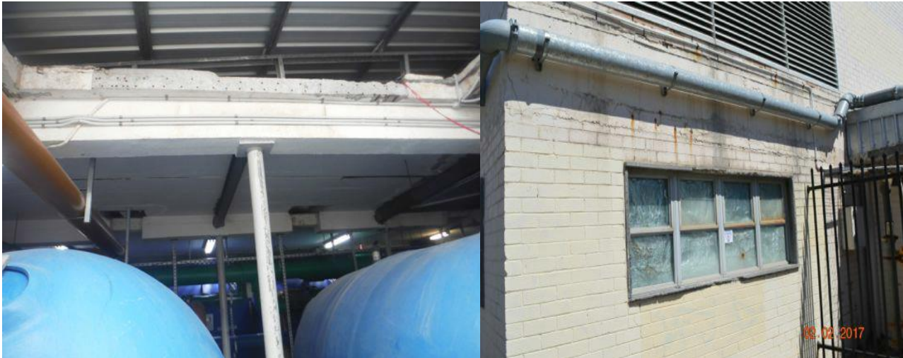
Fig. 2 – Main Plant Room showing internal (left) and external (right) view of perforated and cut slab with fire ring main attached
