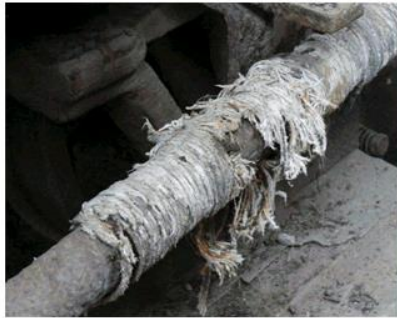
Broken ACM pipe
